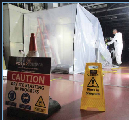
A PORTABLE CONTAINMENT UNIT IS ERECTED AROUND THE WORKS AREA, PREVENTING CROSS-CONTAMINATION OF ANY HAZARDOUS MATERIAL WHILE DRY ICE CLEANING
