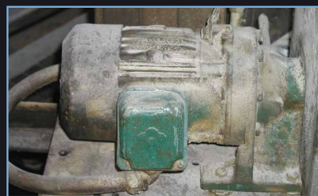
CONTAMINATED ELECTRIC MOTOR BEFORE DRY ICE CLEANING
